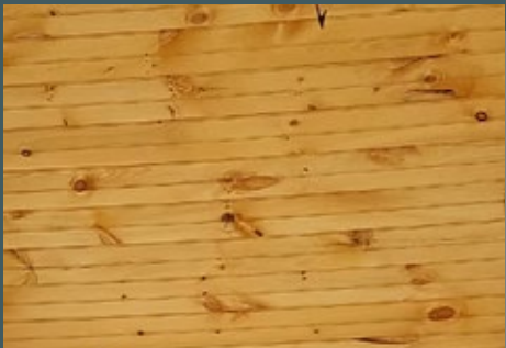
*stained covered rafters
